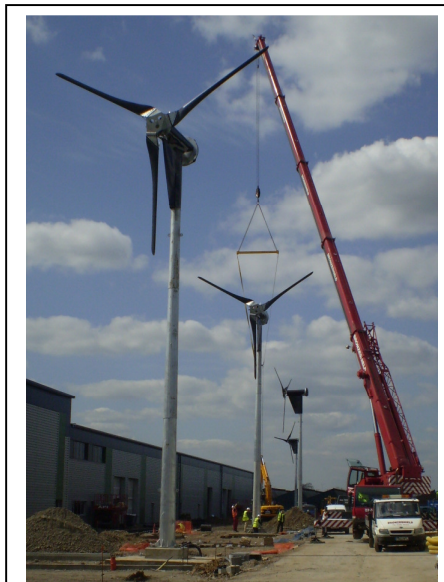
Four 15kW wind turbines at Scotts Road, Southall installed in April 08
