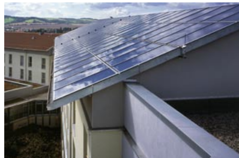
Large-scale solar heating system on the roof of a rehabilitation centre, for hot water, heating and a swimming pool
