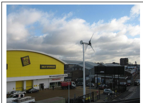
Proven Energy wind turbine installed at Big Yellow Self Storage
